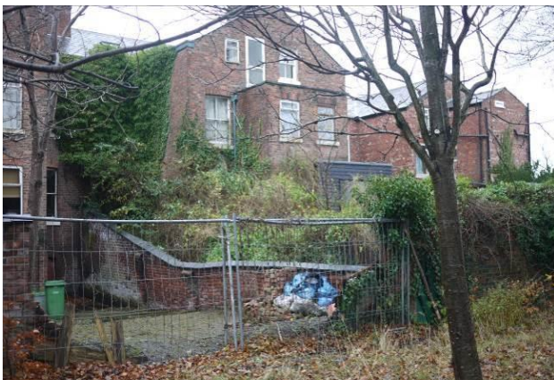
Poor condition of rear elevations of houses backing onto the park
