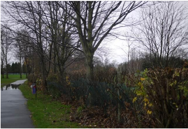
Chain link fencing in a poor condition around the Disc Golf area
