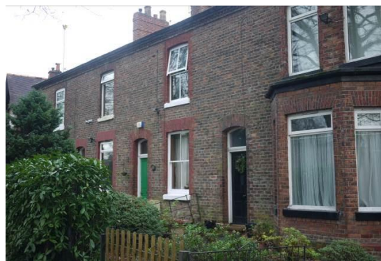
Modern replacement windows in inappropriate uPVC at Longford Cottages
