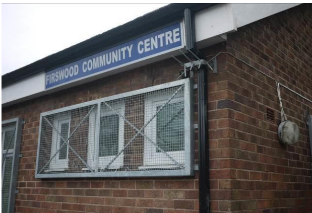
Inappropriate security measures at Firwood Community Centre
