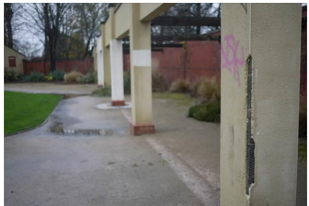
Damage and inappropriate repairs to the Art Deco gardener's store and shelters
