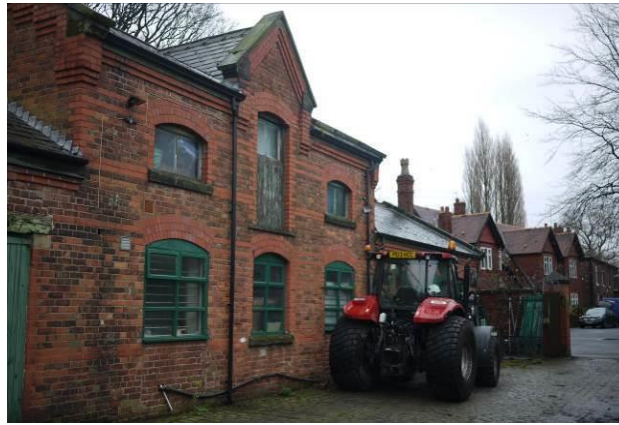
Former stable block in a poor condition
